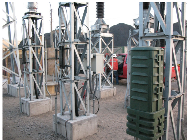
Splice boxes at each of the three phases where the circuit monitoring is terminated.
