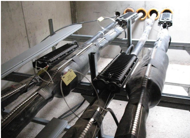
Cable joints and fiber optic splices for each of the phases in the circuit (plus one spare) prior to backfill.
